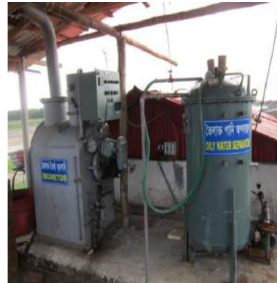
(c) Incinerator and oil/water separator
