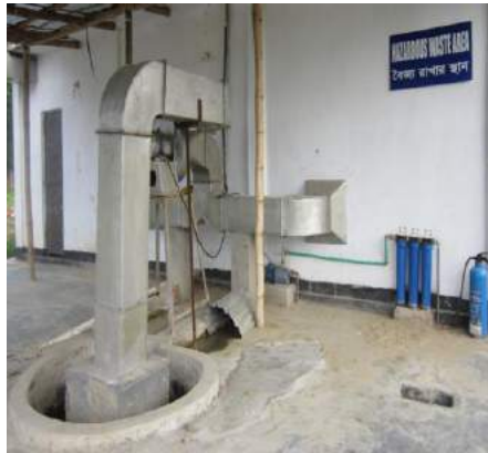
(b) Asbestos treatment facility
